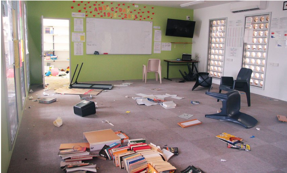
Inside the damaged Don Dale detention facility. Photograph: Helen Davidson for the Guardian
