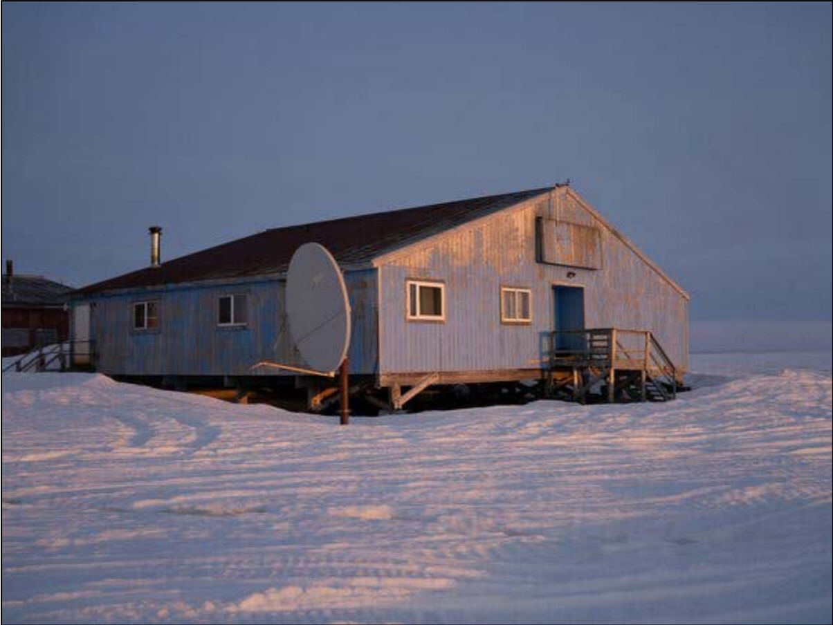
Chefornak's preschool sits on stilts in thawing permafrost. At high tide, water reaches the building, which needs to be moved to safer land.
